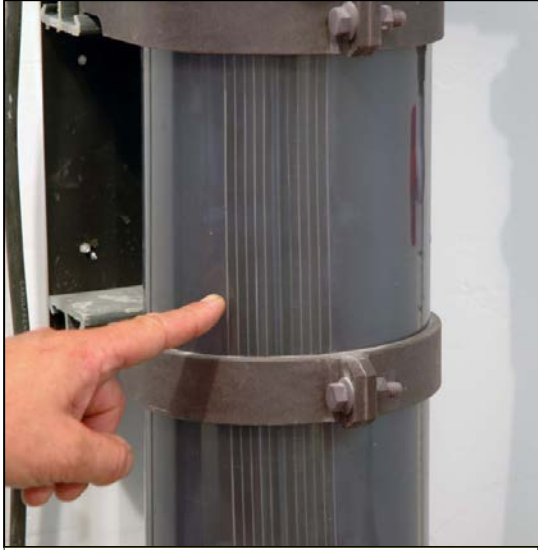
This electrode stack is in excellent condition and does not require cleaning
